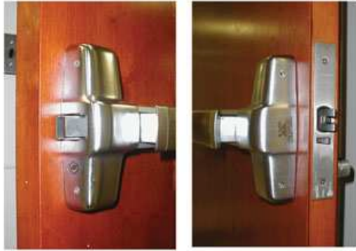
During the site survey process, door hardware details must be noted in order to properly specify electronic door control hardware. The device on the left is a rim-style latch; right, a mortise style.
