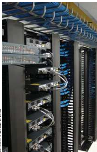
Since electronic access control system (EACS) control panels will most likely interface with the enterprise network, locating them in network equipment rooms throughout the facility makes sense.
